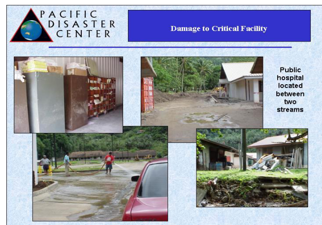
Figure 9: The LBJ Hospital in Tutuila, American Samoa suffered flood damage as a result of the May 2003 floods.
