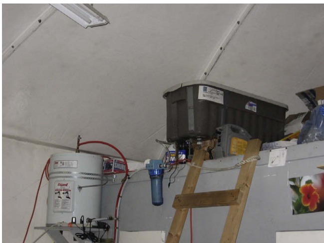
Fig. 2. FMARS main water reservoir, filter, pressure pump and water heater.
